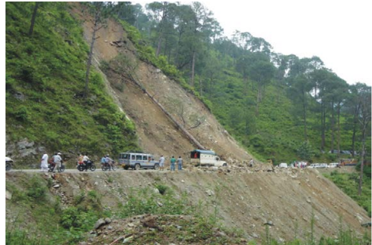
Photo 2: Landslides in Rudraprayag - Guptkashi road
